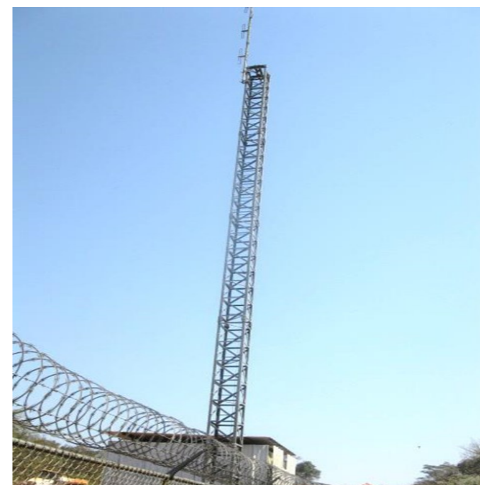
Communication antenna in the Gate(of Severing situated to Lom II, District of Bélabo
