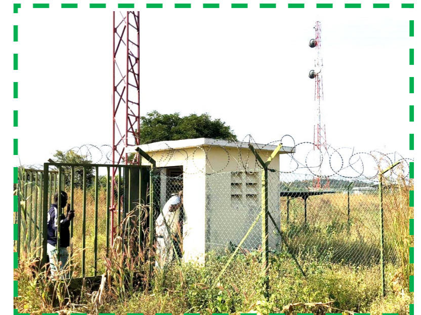
A view of the relay antennas
