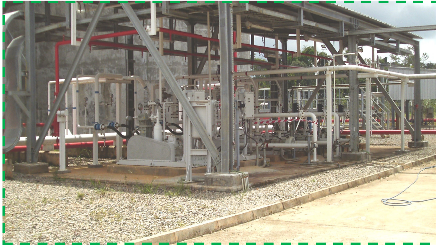
A view of the Bipaga LPG depot
