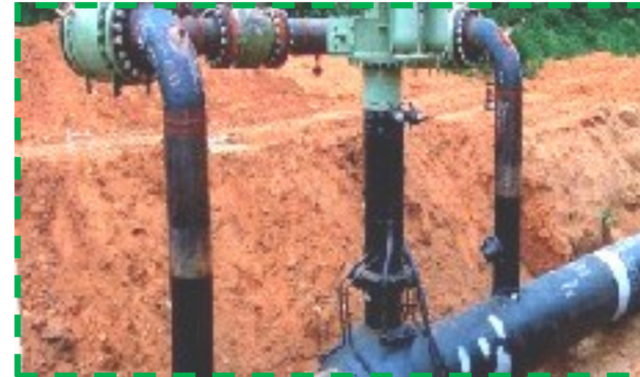
Pump station of Belabo
